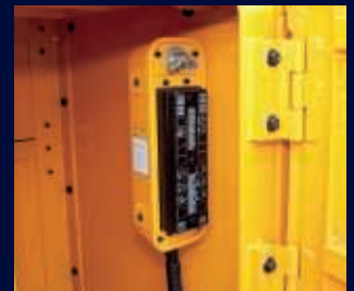
Centralized Fuse Box
